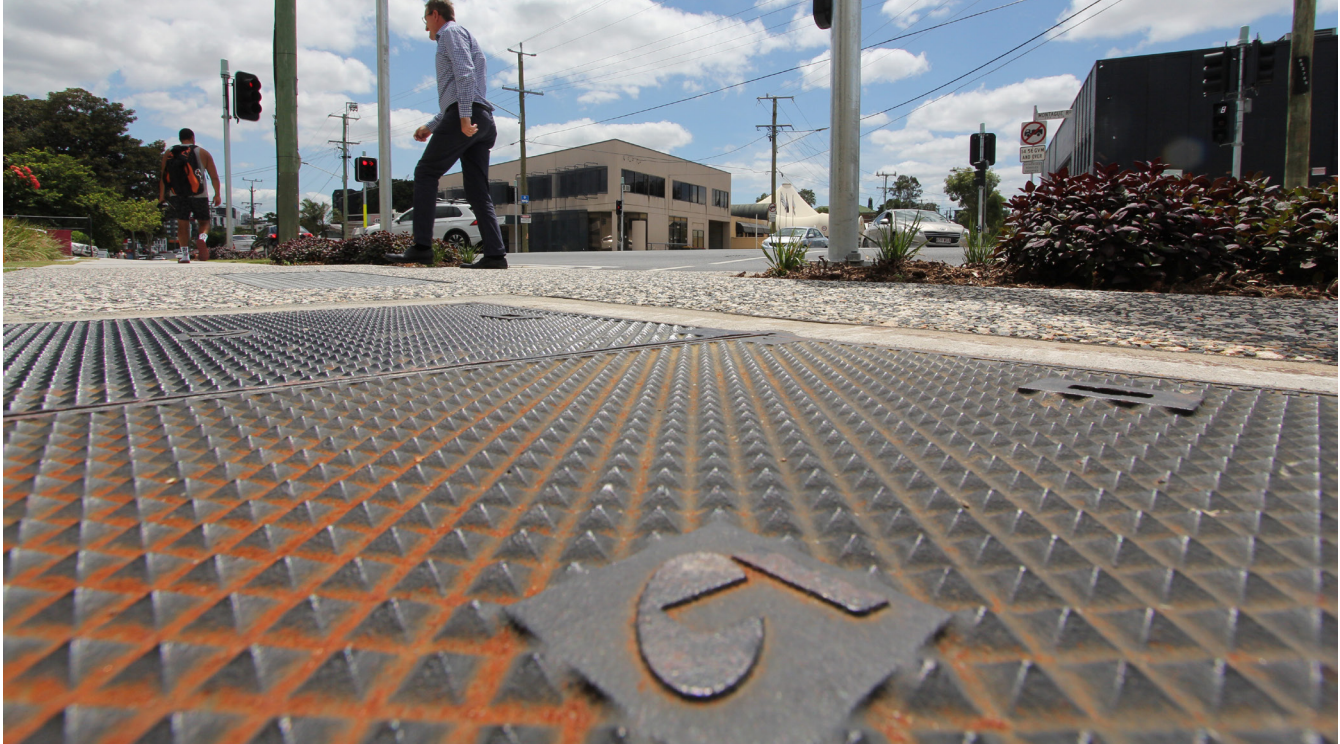
Photography: Ductile cast iron Telstra cover, durable and easily accessible.
