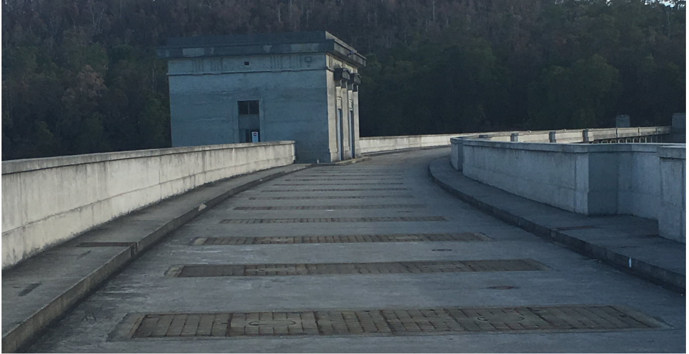
Photography: This shows the covers 25 years after installation, still going strong.
