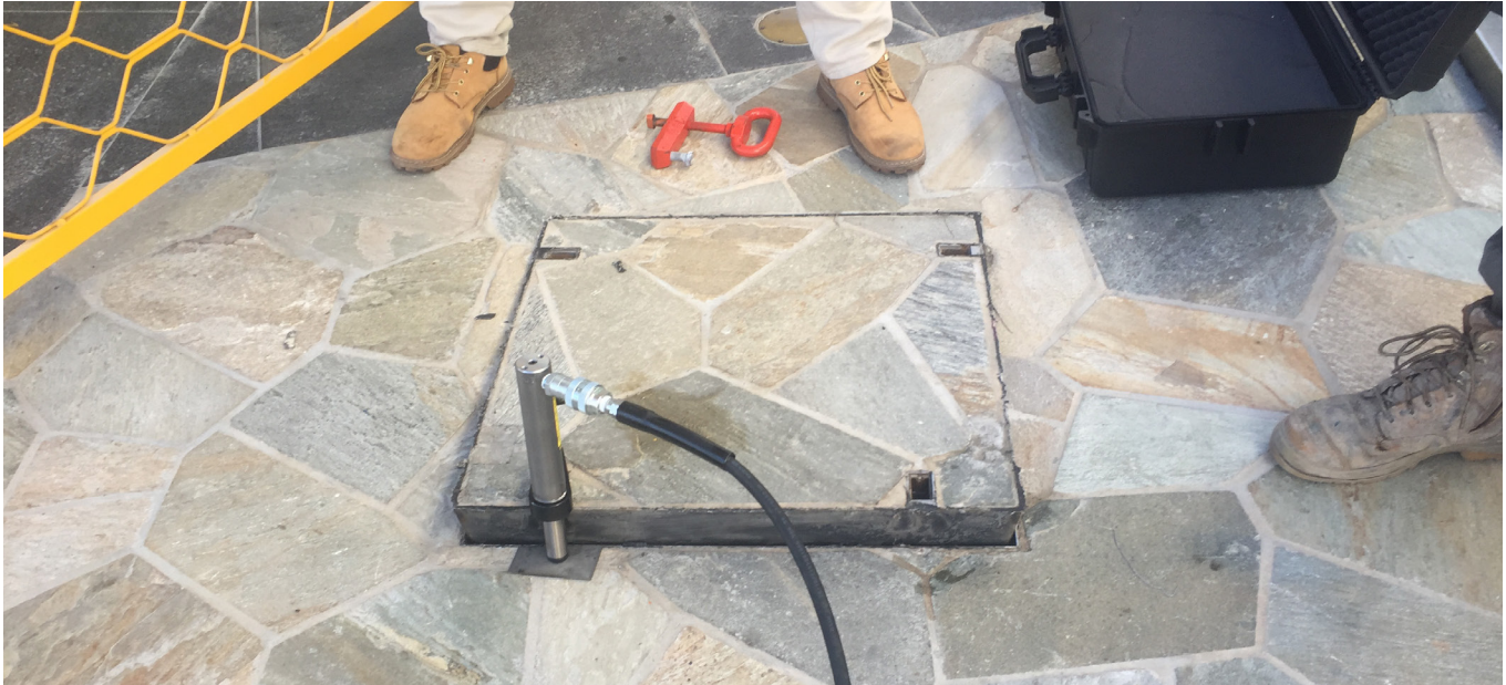
Photography: Paver infill and surrounding concrete undamaged in cover rescue
